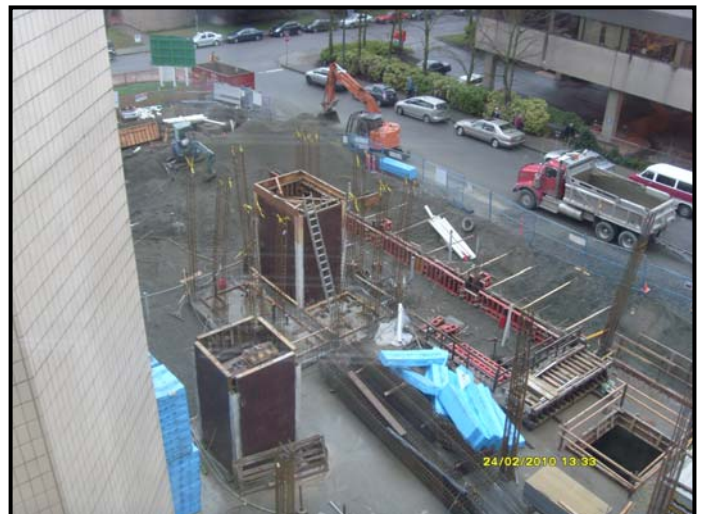
A photo from the fifth floor of the JBRC depicts the overall status of construction – the new building is now at street level.
