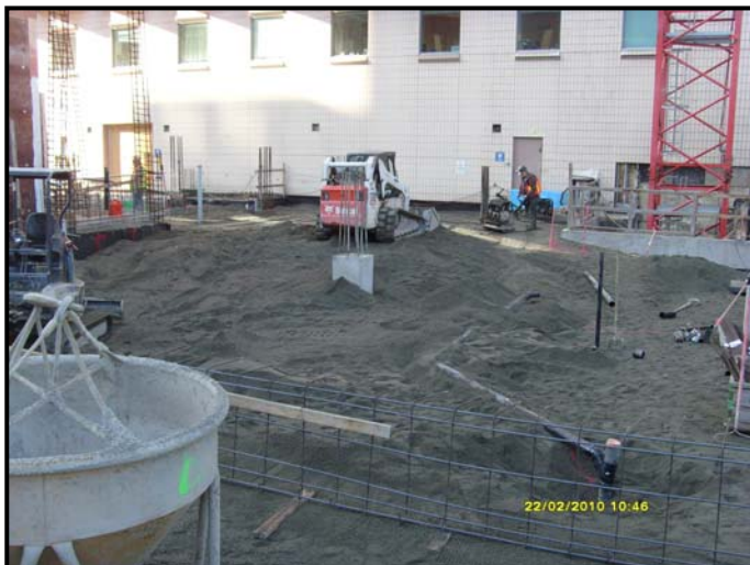
Crews work to compact the structural backfill (background). Reinforcing steel is positioned for the grade beams (foreground).
